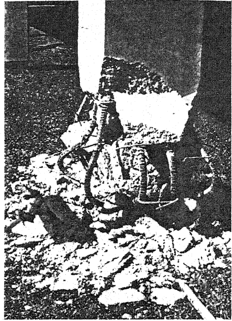
Figure 2. Column failure in Imperial County Services Building in El Centro in October 1979. Column had closely spaced ties immediately below failure.
