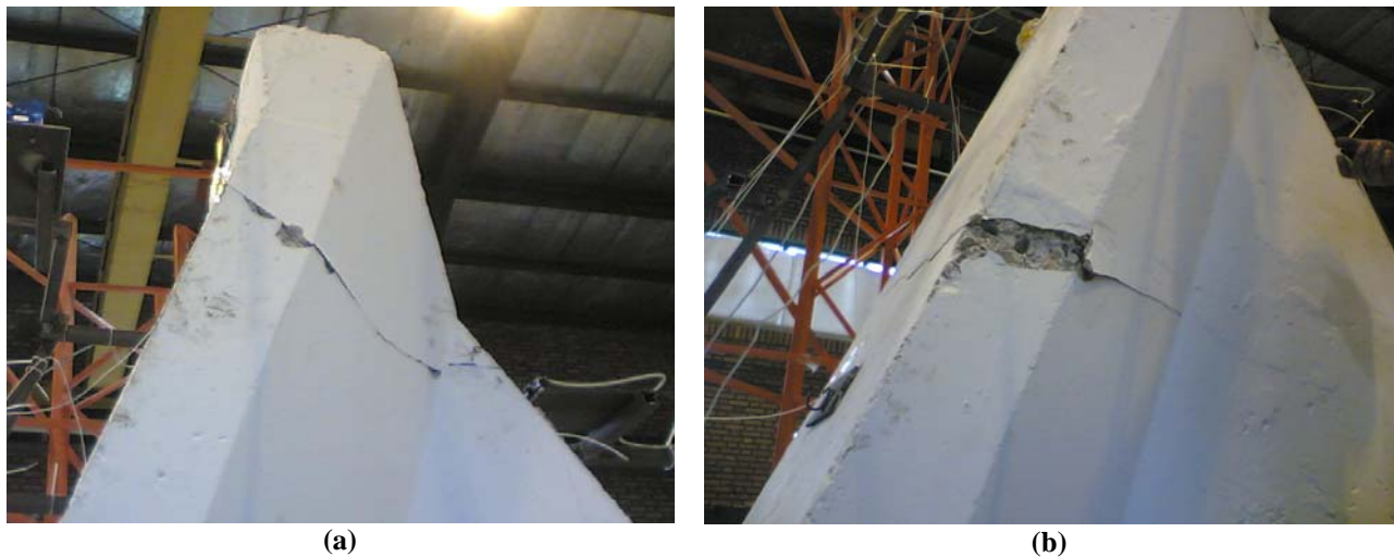
Figure 5: Model cracking pattern: (a) Cracks at the top of the model (b) Cracks at the upstream face of the construction joint no.2
