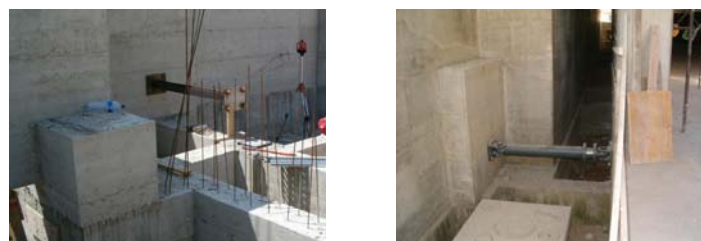
Figure 11 View of a steel spacer and the corresponding spring-damper, before and after the installation of the latter
