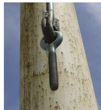
Figure 6: The brittle failure of turnbuckles in the brace of Silakhor village water tank.
