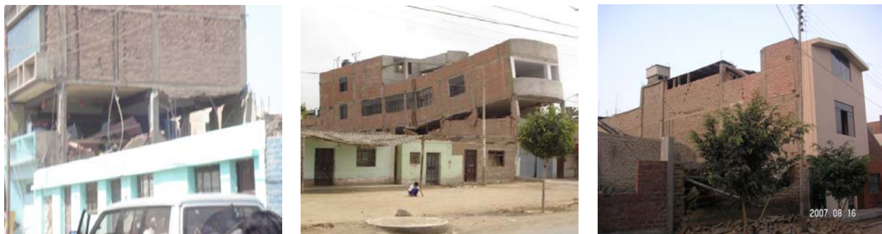
Figure 11. Left and center: damage in buildings with concrete frames filled with tubular bricks Right: damage in building with tubular masonry walls, lack of confinement.
