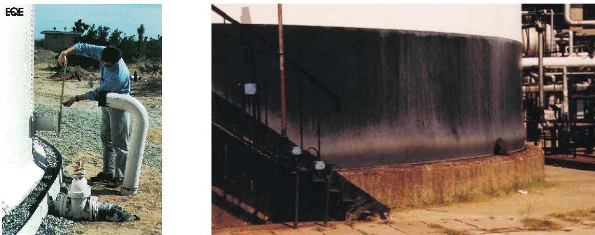
Figure 1 (left) Example of I/O pipe failure ( http://www.eqe.com ); (right) Elephant Foot Buckling damage in Turkish plant. (Kocaeli, 1999, Turkey; Saatcioglu et. al. 2001)
