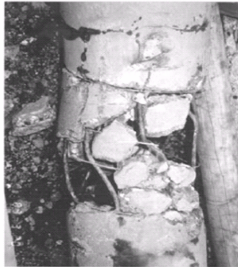
Figure.1 Damage to pile by 2m of lateral ground displacement during 1964 Niigata earthquake (Yoshida et al.1990)
