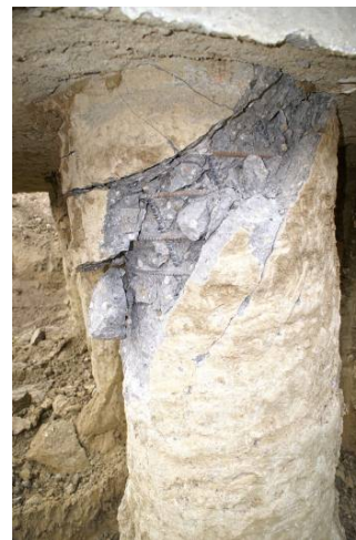
Figure 11: Concrete spalling at a pile
