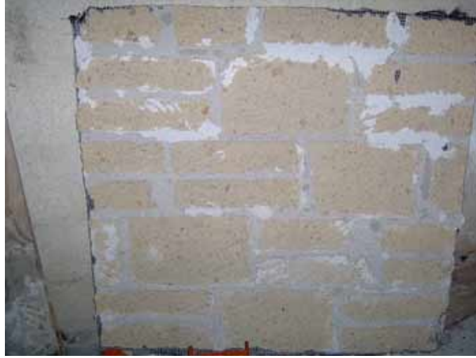
Figure 12: FRP plate peeled off after interface delamination
