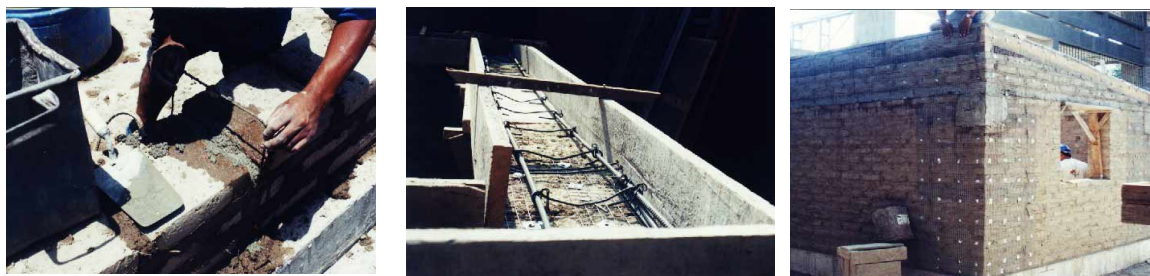
Fig. 7. Some structural improvements in the new adobe houses: wire connector in joint (left), collar beam (middle), and shear key (right).
