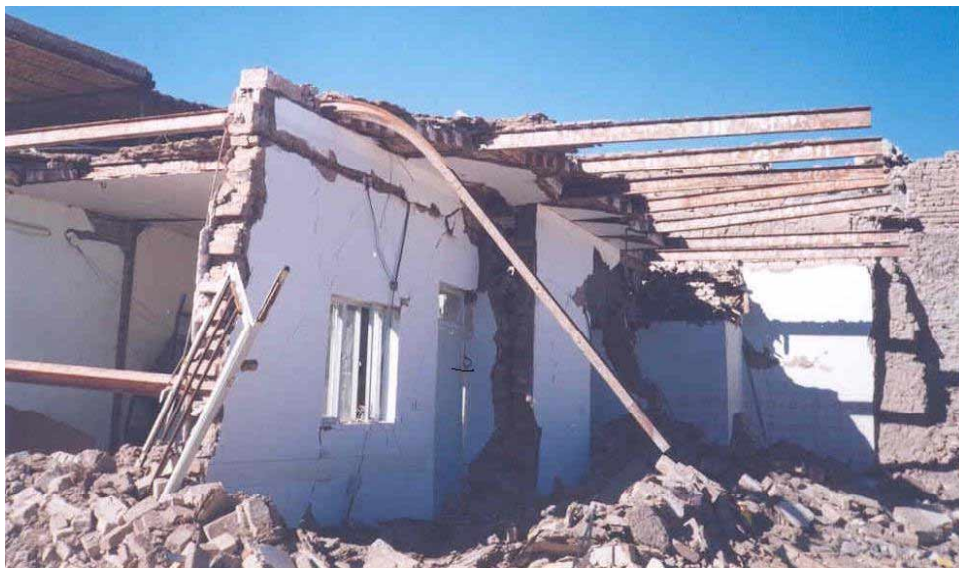
Fig. 1 Damage to the traditional jack arch slab during Bam earthquake of 2003
