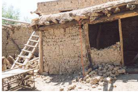
Figure 2: A typical traditional building with wooden beams and columns in western Iran after the 2002 Avaj's earthquake.
