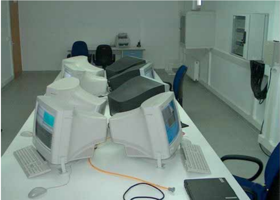
Fig. 5: Main data Center.
