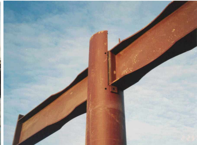
Photo 1b: Bent Plate Closure on Girder Web.
