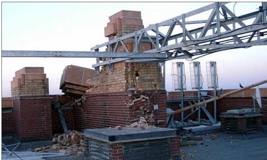
Fig. 3: URM roof pinnacle damage shown with temporary bracing.
