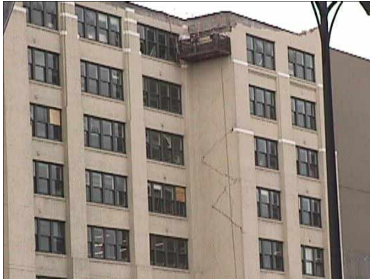
Fig. 8. Starbucks Center building damaged URM parapet and exterior cladding, USGS [5].
