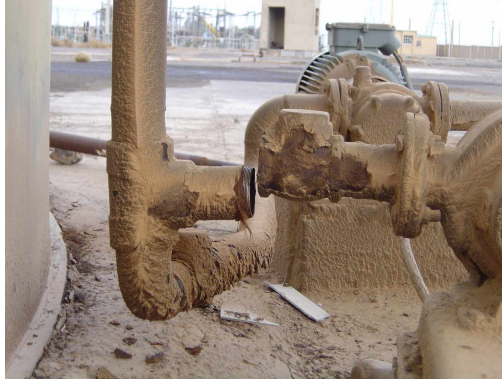
Figure 1- Failure of Rigid Piping Due To The Bam Near-fault Earthquake
