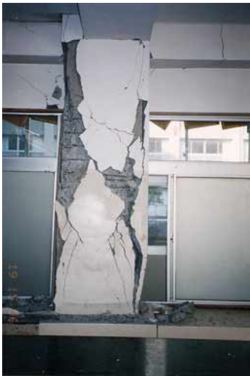
Damage class IV: Exposed rebar without buckling or fracture
