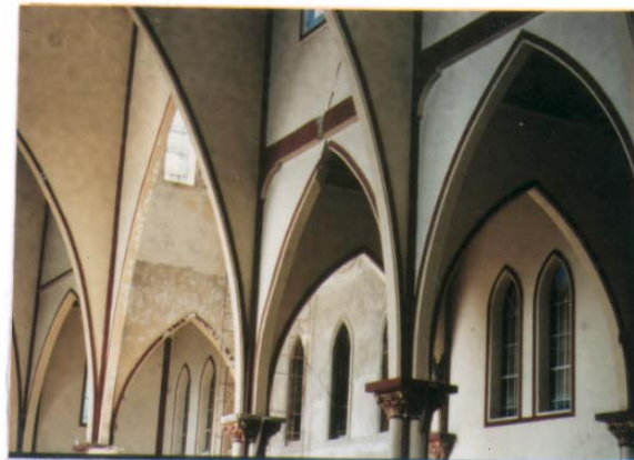
Photo 10. San Antonio Church. Discontinuity in the zone of the Presbytery
