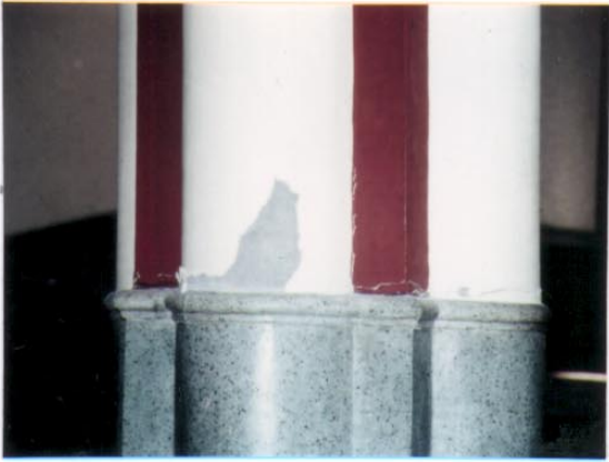
Photo 13. San Antonio Church. Cracking at the base of the central column.
