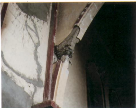
Photo 11. San Antonio Church. Severe damage at the column-arch joint.
