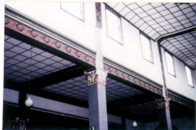
Photo 6. Plaster fell off from the top of column in Balbanera Church.
