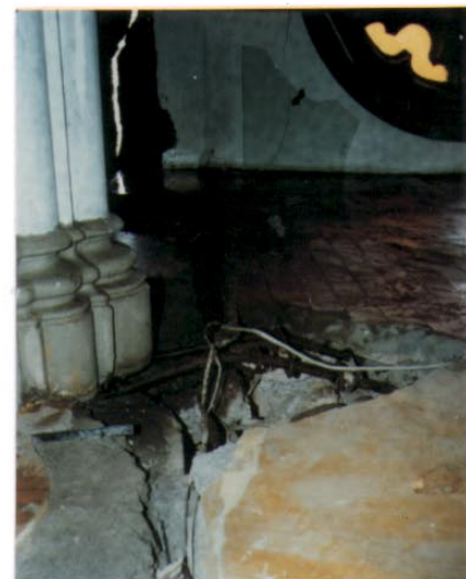
Photo 18. San Jose Church. Severe damage in the section between the Chorus and the Central Nave.
