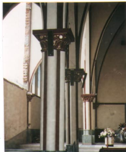
Photo 12. San Antonio Church. Lack of verticality of central column.
