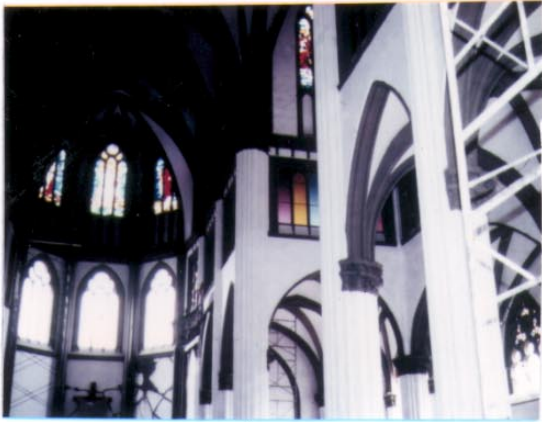
Photo 15. San Jose Church. Beam without continuity to the Presbytery
