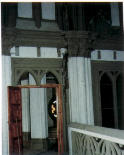
Photo 17. San Jose Church. Separation of the structures of Chorus and Central Nave.
