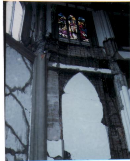
Photo 16. San Jose Church. Fracture of short columns at the Presbytery
