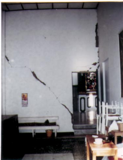
Photo 5. Great cracks in the Presbytery of Balbanera Church.
