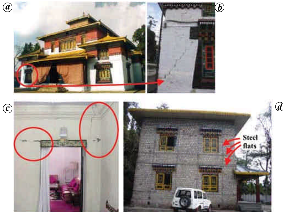
Figure 3. Performance of masonry structures at Gangtok. a, b , Wide shear and vertical cracks in masonry walls at corners and near openings in Enchey Monastery. c , Numerous cracks near door/window openings were observed at Raj Bhavan. d , Good performance shown by retrofitted Archive building (arrows show steel flats used to retrofit the building after the 1988 Bihar–Nepal earthquake).
