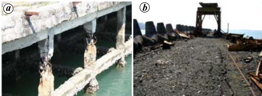
Figure 6. a , Severe corrosion led to damage of columns of approach jetty at Rangat Bay Harbour in Middle Andaman. b , Rangat Bay Harbour in Middle Andaman, longitudinal cracks on top of the breakwater.
