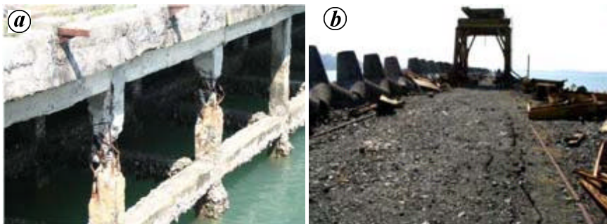
Figure 6. a , Severe corrosion led to damage of columns of approach jetty at Rangat Bay Harbour in Middle Andaman. b , Rangat Bay Harbour in Middle Andaman, longitudinal cracks on top of the breakwater.
