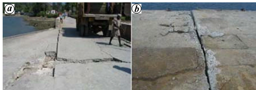
Figure 3. Pounding damage to jetties in Middle Andaman (a) at the junction of solid jetty and RC piled approach jetty at Rangat and (b) in the berthing jetty at Mayabandar.
