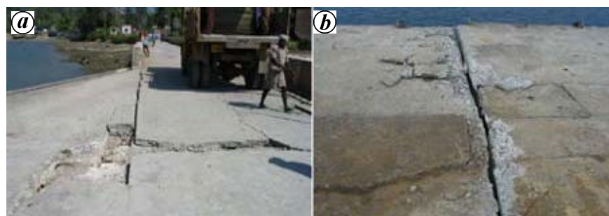
Figure 3. Pounding damage to jetties in Middle Andaman (a) at the junction of solid jetty and RC piled approach jetty at Rangat and (b) in the berthing jetty at Mayabandar.
