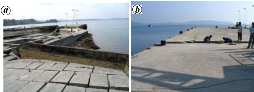
Figure 5. a , Damaged side bund of slipway at Mayabandar Harbour in Middle Andaman due to liquefaction of soil. b , A portion of the berthing jetty at Diglipur Harbour sunk due to failure of piles. This portion of the jetty cannot be approached by the vehicle for loading/unloading of goods.
