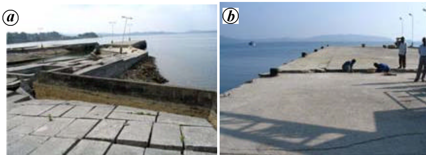
Figure 5. a , Damaged side bund of slipway at Mayabandar Harbour in Middle Andaman due to liquefaction of soil. b , A portion of the berthing jetty at Diglipur Harbour sunk due to failure of piles. This portion of the jetty cannot be approached by the vehicle for loading/unloading of goods.
