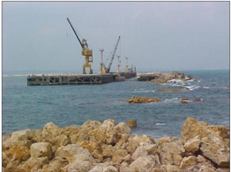
Figure 11. Shortage of appropriate construction material forced the use of porous coral stones from local quarries for building the breakwaters. The stones were easily uplifted during the tsunami and breached a large segment of the approach to the RC jetty at Hut Bay (photo: C.V.R Murty).
