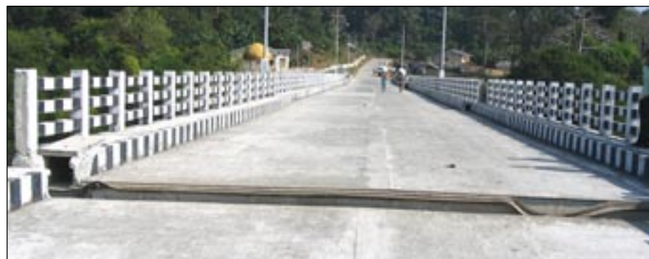
Figure 10b. Detail of the bridge deck showing lateral and vertical displacement due to shifting of the decks on their neoprene bearings (photo: Durgesh C. Rai).
