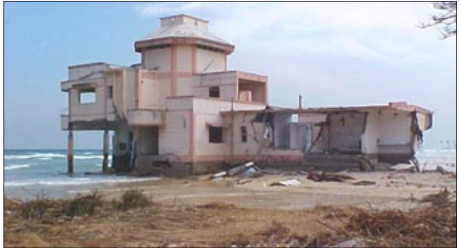
Figure 3. RC frame building (MES Inspection Bungalow) now stands in water on the eastern coast of Car Nicobar Island (photo: C.V.R. Murty).
