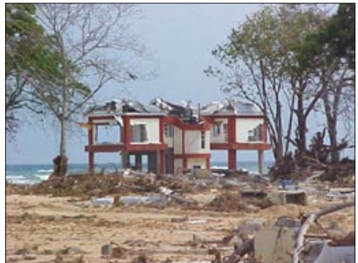
Figure 7. Shore-front building on Car Nicobar Island was inundated by the waves, but the frame resisted the wave effects (photo: C.V.R. Murty).
