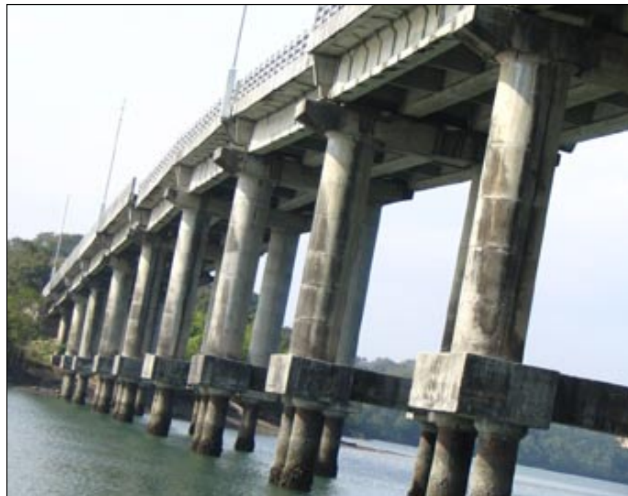
Figure 10a. Chengappa Bridge over Austen Strait was rendered dysfunctional by displacement of the middle spans (photo: Durgesh C. Rai).
