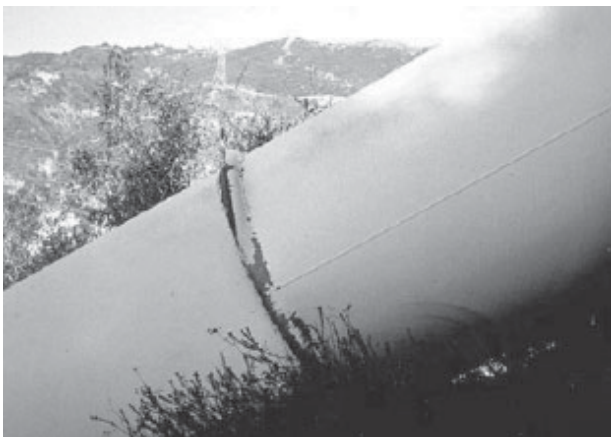
Figure 3: Locally buckled steel gas pipeline in the compression zone at North slope of Terminal Hill in 1994 Northridge earthquake. (EERI, 1995)
