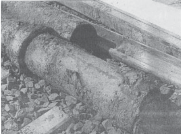
Figure-6: Failed cast iron pipe due to failure of bell and spigot joint at Navlakhi port due to lateral spread in 2001 Bhuj earthquake (ASCE, 2001)
