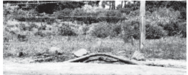
Figure 4: Beam buckling of a water pipeline made of iron. (USGS Photo Library)
