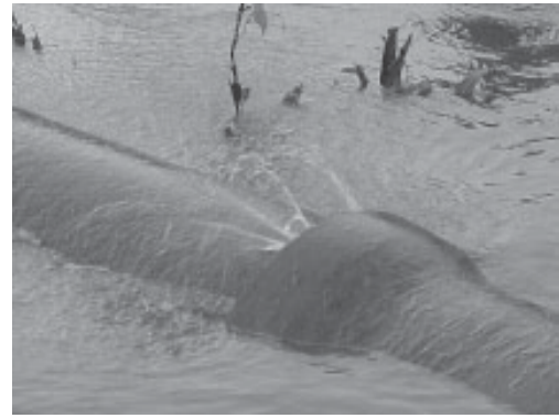
Figure-8: Leaking at bell and spigot joint of water supply pipeline due to bending at Shippy Ghat, Port Blair in M9.0 Sumatra earthquake of 2004 (Photo: Suresh R Dash)
