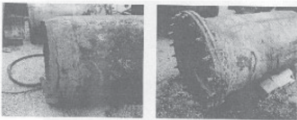
Figure- 7: Flanged joint pipe failure. (ASCE, 1997)
