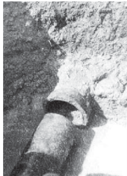
Figure-5: Axial pull-out at the joint of a water supply pipeline at Tangshan East Water Works in Tangshan Earthquake 1976 (EERI, 2004)
