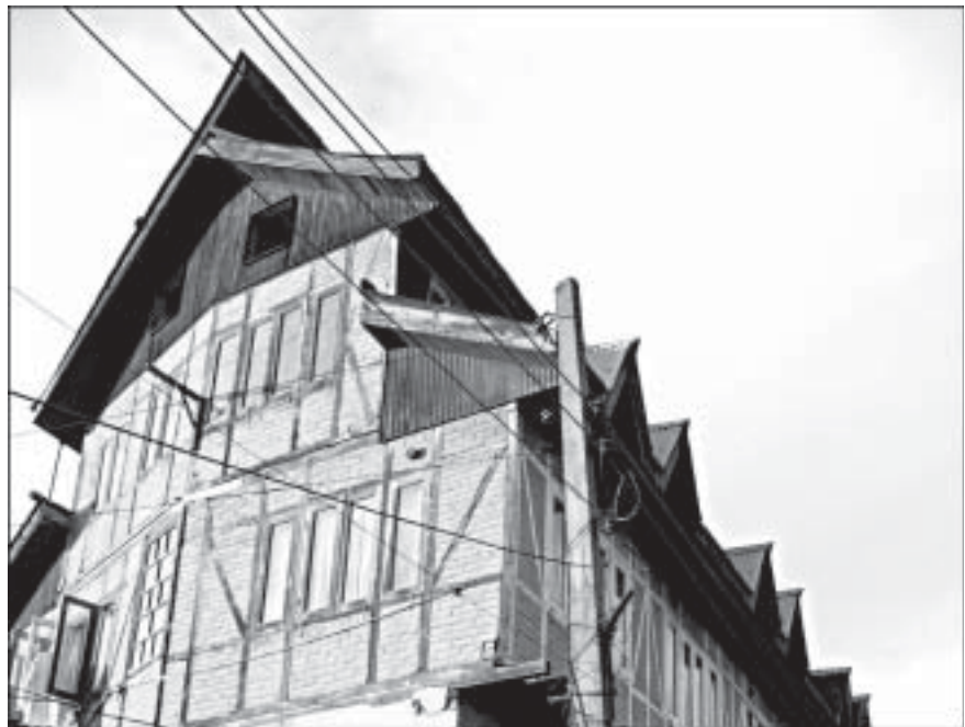
Fig 1 Dhajji-dewari system of timber-laced masonry for confining masonry in small panels withstood the earthquake without serious damage
