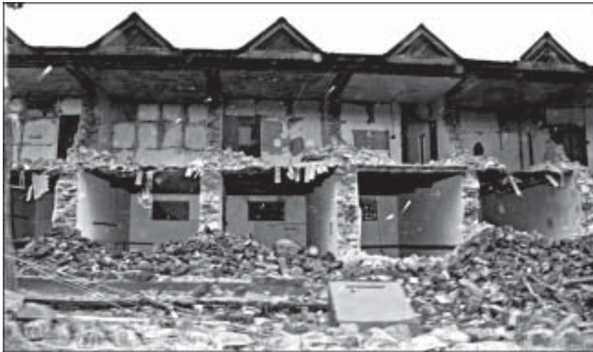
Fig 3 Collapse of stone masonry walls
