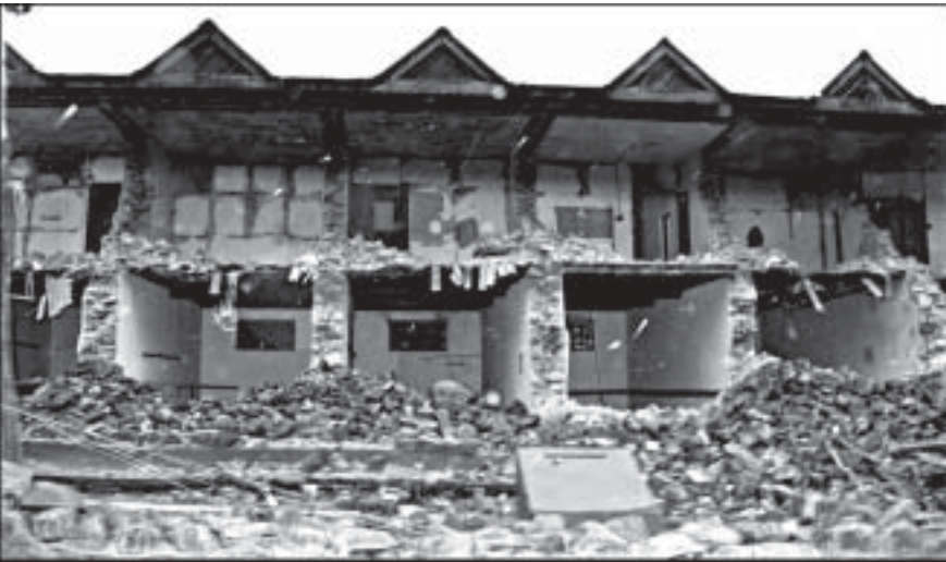
Fig 3 Collapse of stone masonry walls
