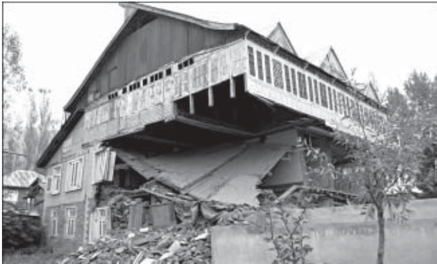
Fig 2 Timber frame and timber-laced masonry held on as stone masonry walls in lower storeys collapsed
