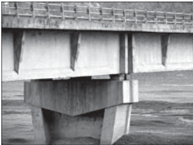
Fig 4 Prestressed concrete girder bridge lacks restrainers to prevent unseating during earthquakes at this bridge in zone V
