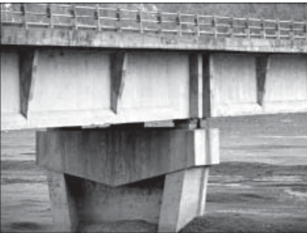
Fig 4 Prestressed concrete girder bridge lacks restrainers to prevent unseating during earthquakes at this bridge in zone V
