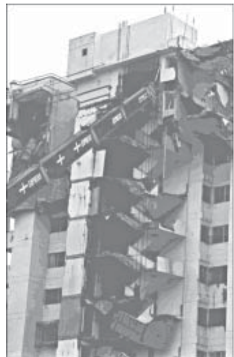
Fig 2 Failure of signboard in Bhuj earthquake, 2001 (Photo credit: Alok Goyal 10 )
