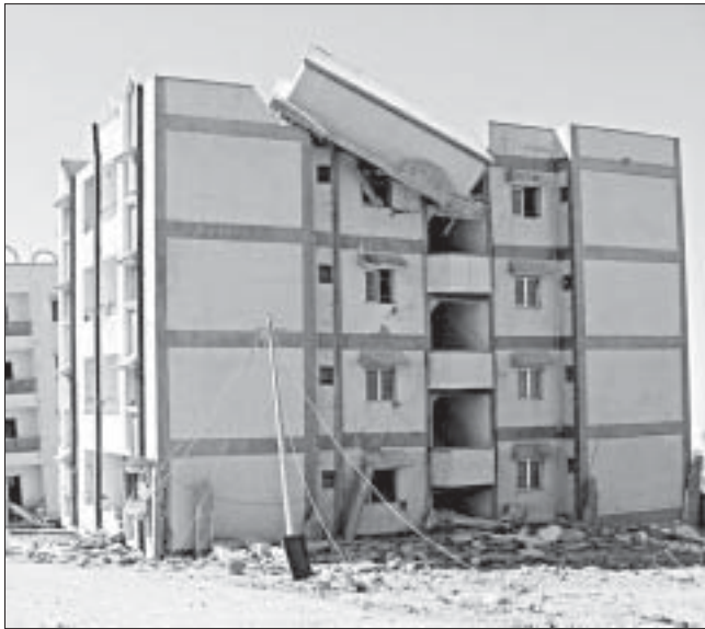
Fig 1 Failure of overhead tank in Bhuj earthquake, 2001 (Photo credit: C.V.R. Murty 10 )
