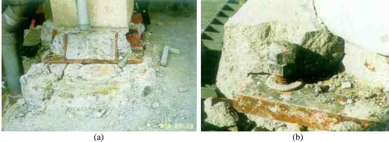
Figure 2: Column foundation damage: (a) Crushing of concrete pedestal of column-foundation joint due to pounding of base plate on the pedestal, and (b) Pull-out of anchor bolts and crushing of concrete pedestal at column-foundation joint during 1995 Kobe earthquake (AIJ, 1995). Pounding of base plate and pull-out of anchor bolts implies significant uplift of the base plate.
