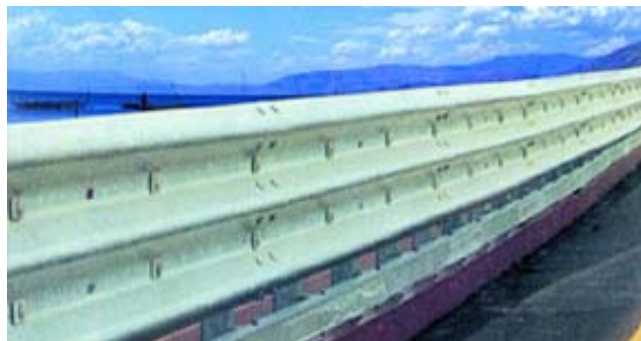
Figure 10: Steel Guardrail Systems (Source: www.kirby-india.com , 2004)
