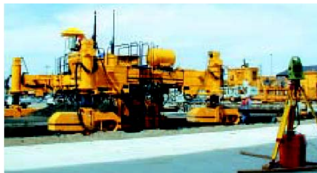
Figure 12: Automatically guided slip-form paving machine and on-ground monitoring systems for transferring information from ground to machine. (Source: www.leica-geosystems.com , 2004).
