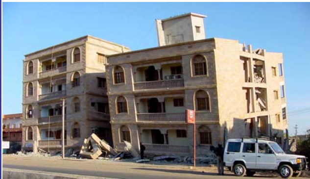
(b) 2001 Bhuj Earthquake
