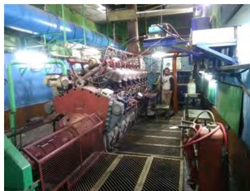
ALCO251 locomotive engine at RDSO Lucknow for Methanol Conversion
